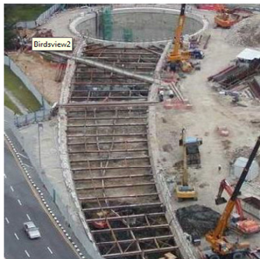
(a). Before collapse
