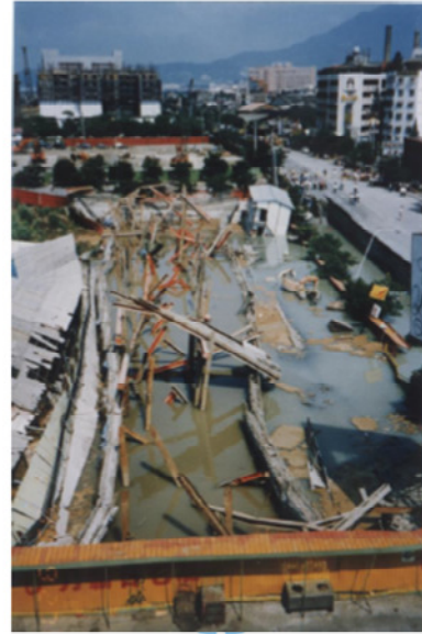
Fig. 3 Photo of Rebar Broadway Excavation Failure (Private document)
