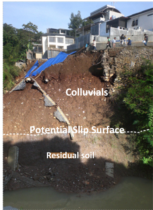
Fig. 8 Photo of the potential slip surface at the interface of fill and residual soil.
