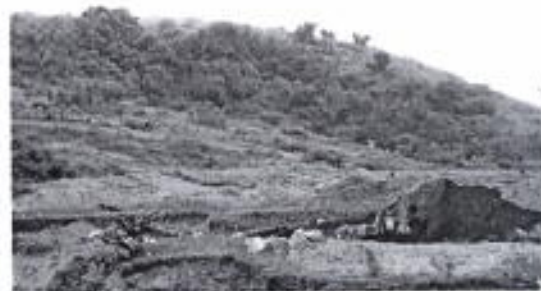
An Excavator on an Infrastructure Project in West Java. Creator: Yulius Purwadi Hermawan. This image is licensed under Creative Commons License .
