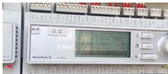
Gambar I. 1 Panel Mesin Chiller HVAC Phase 2
