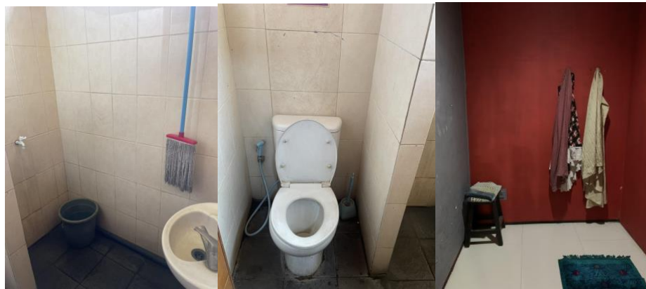
Gambar 1.1 Kondisi Toilet Sate Taichan Goreng Tamansari Bandung
