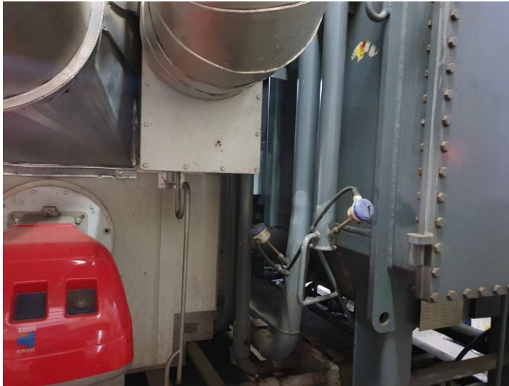
Gambar I.5 Mesin AC Absorption Chiller
